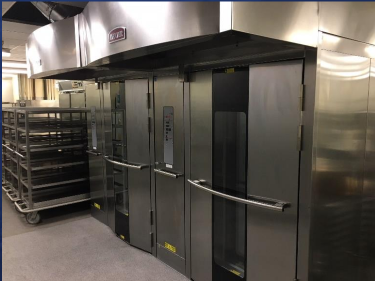
Installed 2 Rotating Ovens
